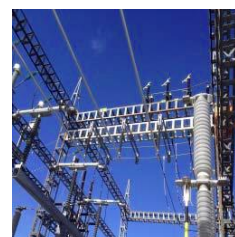
Pilot installation Vattenfall, SE AIS 3rd party NCIT, 670, 630, 615series
