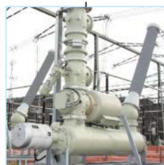
Pilot installation Laufenburg, CH GIS NCIT, 670series, REB500
