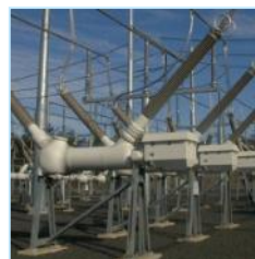
Pilot installation Braemar, AU GIS NCIT, 670series
