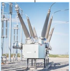
Pilot installation US DTB with FOCS, SAM600, 670 series
