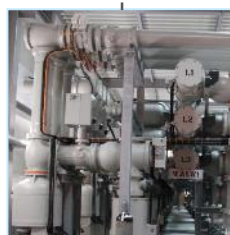
Pilot installation CH GIS NCIT, 670series, 3rd party
