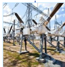
Real installation Braemar, AU* GIS NCIT, 670series, REB500
