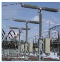
Pilot installation SvK, SE DCB with FOCS, 670series
