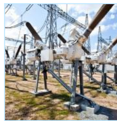
Real installation Millmerran, AU GIS NCIT, 670series, REB500
