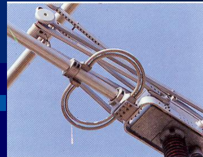
Tubular conductor with expansion clamp.
